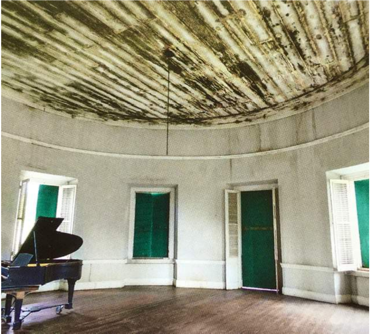
Damage to the Whim Museum ceiling after Hurricanes Irma and Maria in 2017. (Photo courtesy of Michael Connors)
