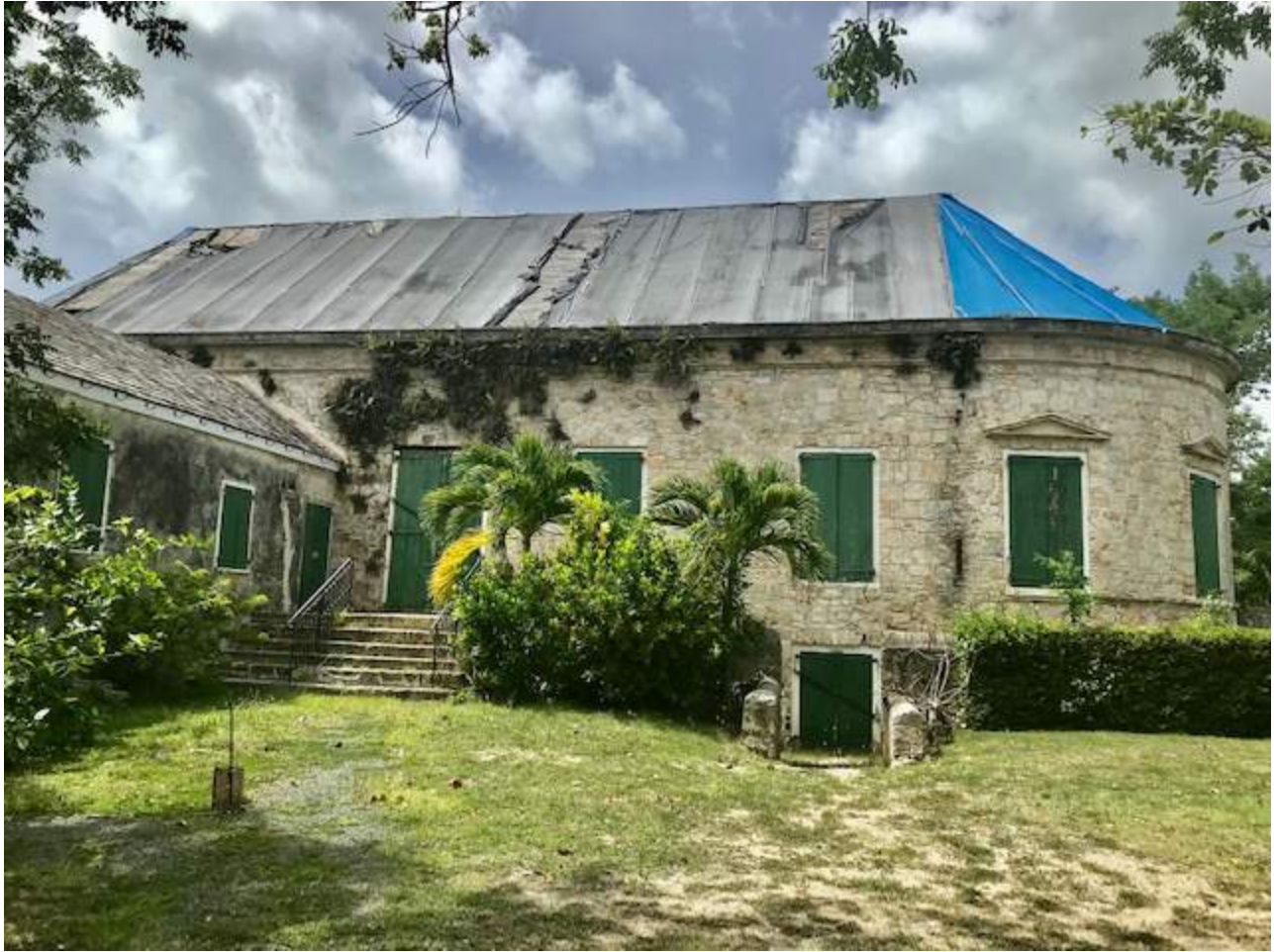
South view of Whim Museum hurricane damage in 2017. (Photo courtesy of Michael Connors)
