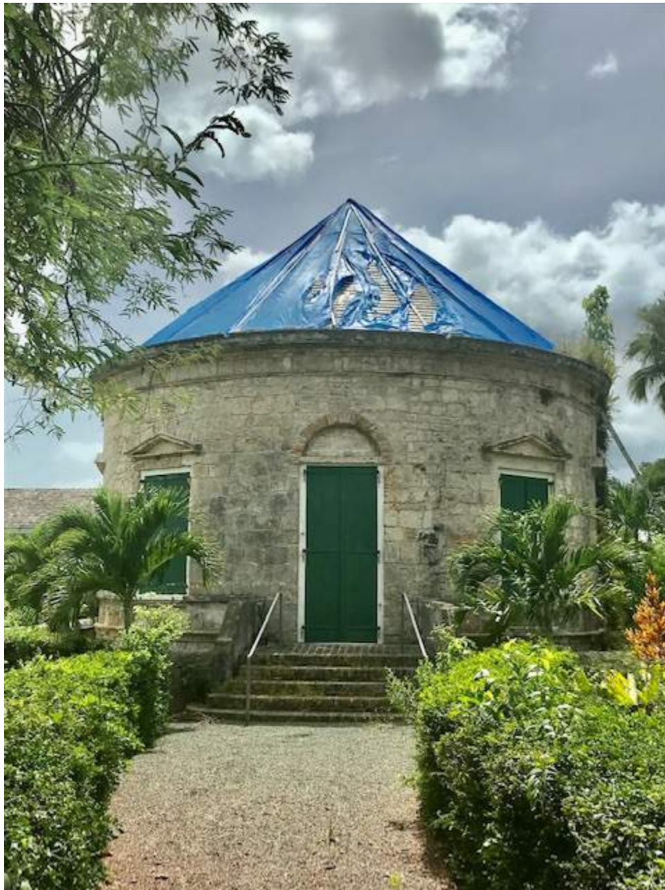
Whim Museum roof damage from 2017 hurricanes. (Photo courtesy of Michael Connors)
