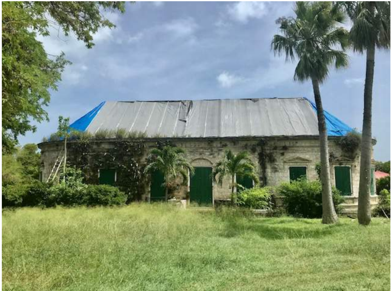
Hurricane damage on the north side of Whim Museum from 2017. (Photo courtesy of Michael Connors)
