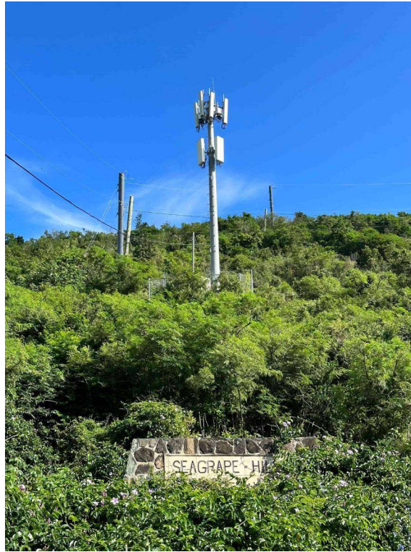
Figure 2. Cell tower at Seagrape Hill on STJ. It is common to place towers at elevated locations to avoid interference from hills, trees, and built structures (Federal Communications Commission 2020).
